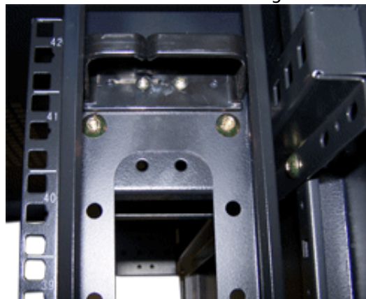
Fastened cable manager
